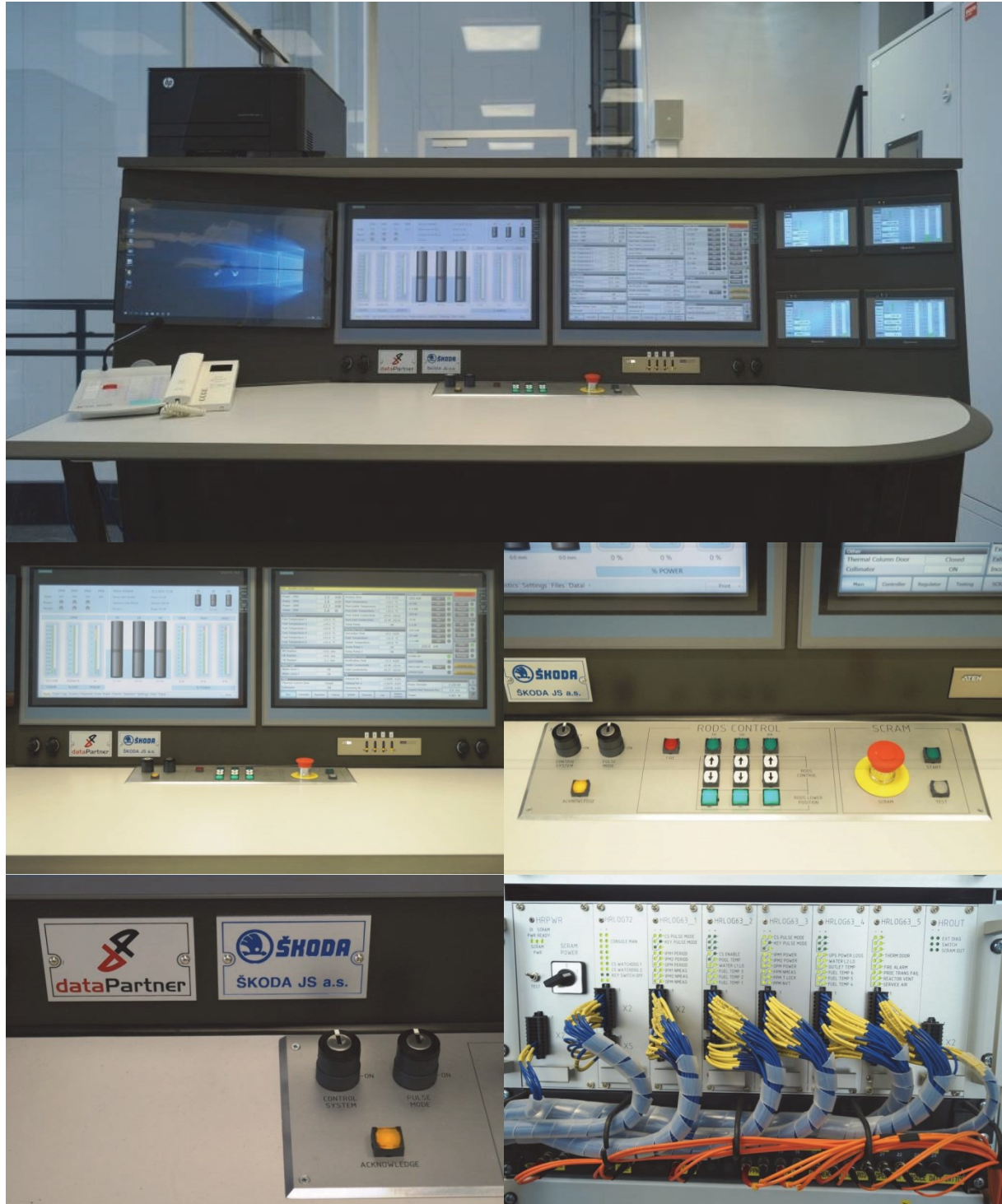
The new I&C system of the TRIGA Mark II Reactor Vienna, November 2015
