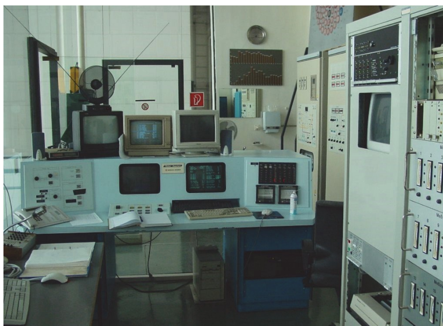
Digital Reactor Instrumentation 1992
